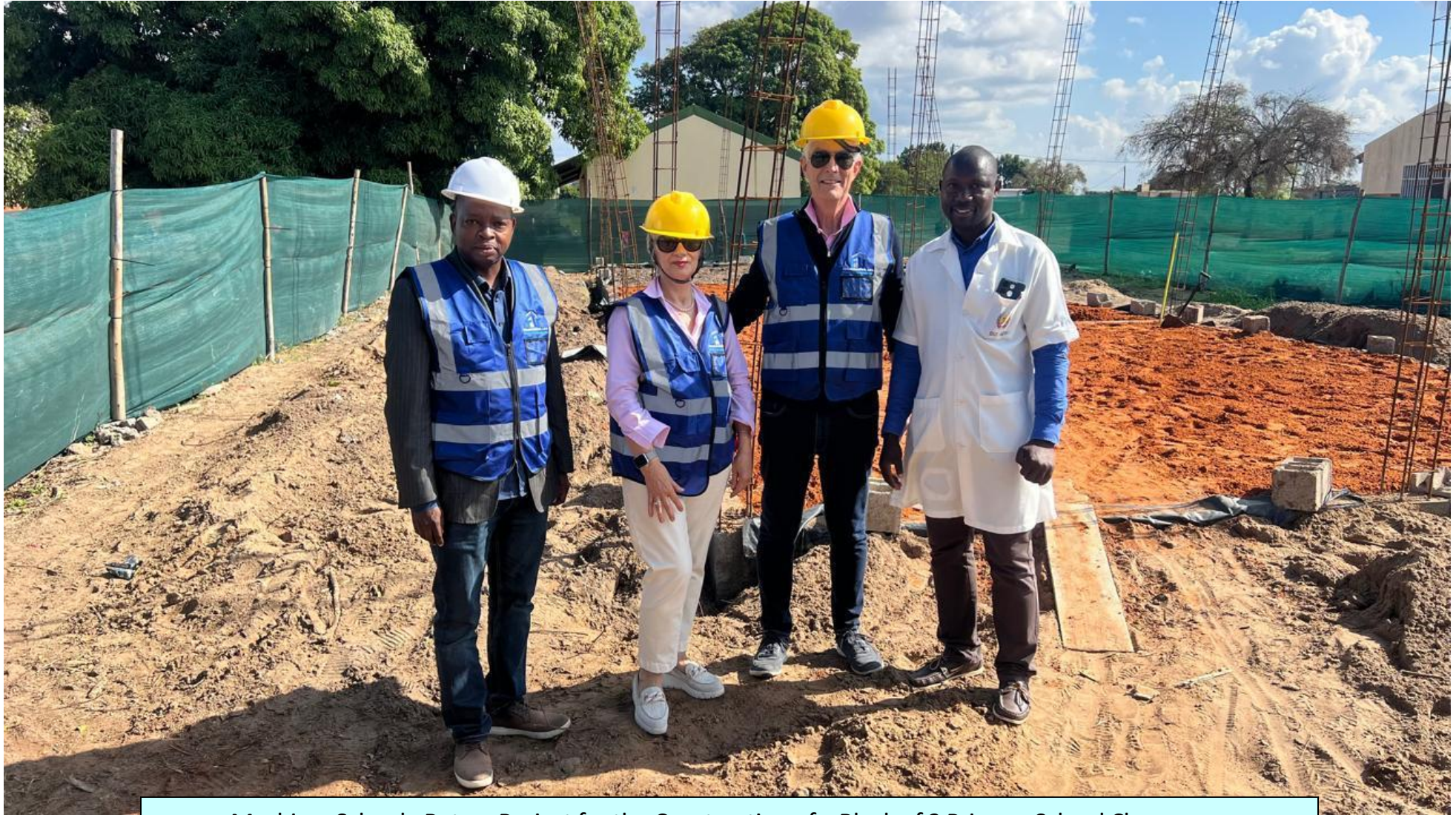
Machisso School - Rotary Project for the Construction of a Block of 3 Primary School Classrooms
